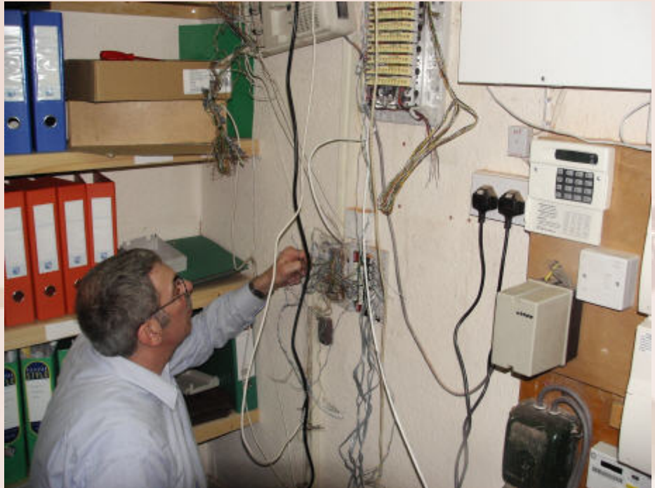
Installing the new phone system at Fox Evans. HBT Communications estimates it will reduce landline bills by 20 to 30%, cut mobile bills by 12% and halve electronic communication costs.
